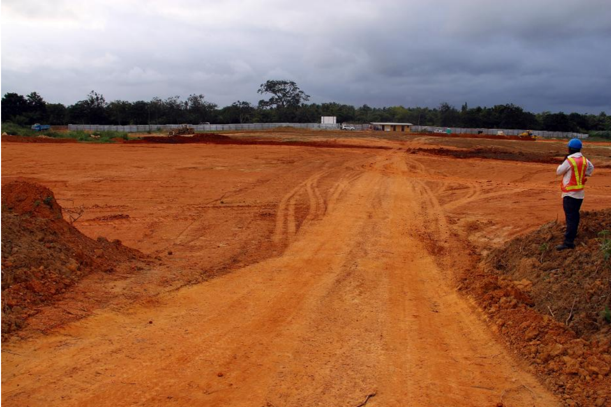
Construction of Oilfield Logistics Base begins at Genesis' 43-acre (174,000m 2 ) site in Takoradi
